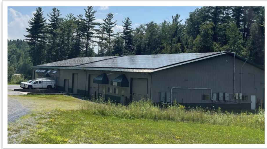
Solar power generation at the South Road Enterprise Area
