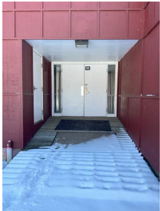
Exterior egress ramp not compliant
