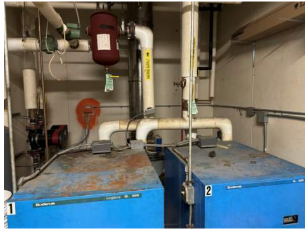
Oil boiler—near end of useful life
