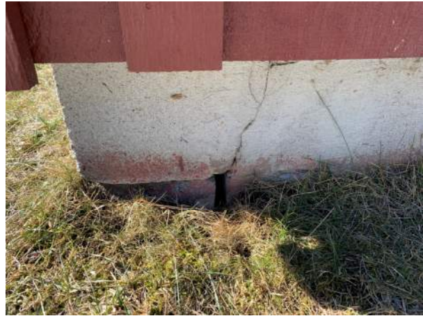
Cracks in exterior CMU foundation wall
