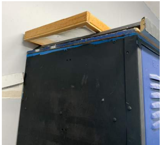
Corridor lockers in poor condition
