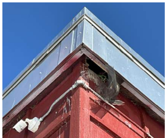
Displaced soffit vent
