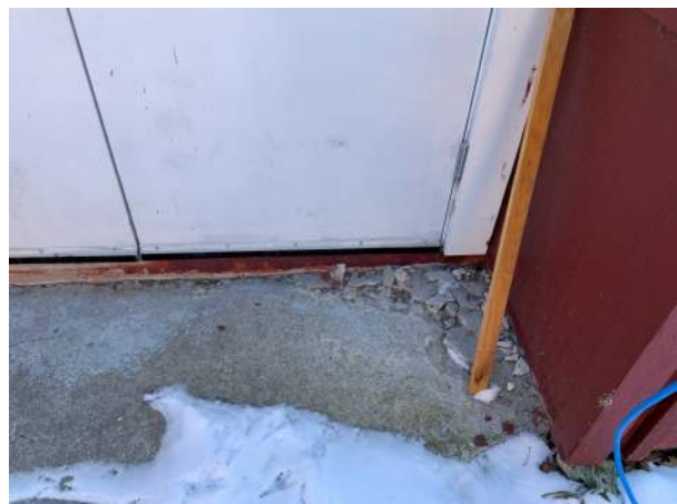
Spalling of exterior concrete slab
