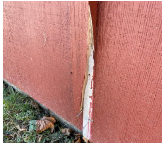
Damaged exterior siding trim
