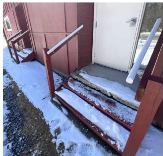
Classroom egress doors—not accessible
