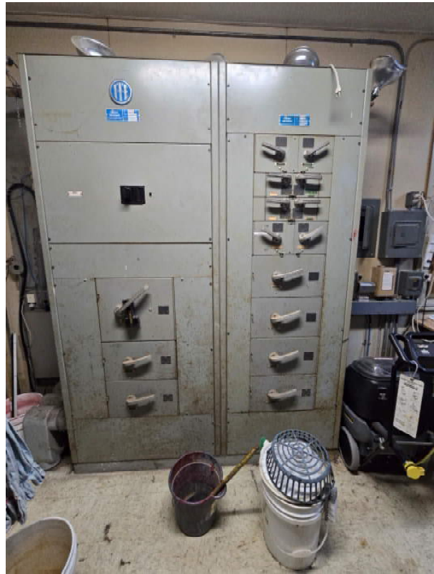
Original electrical gear—nearing end of useful life
