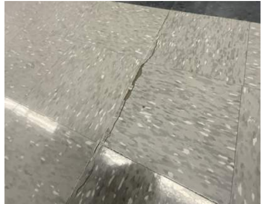
Cracked VCT flooring
