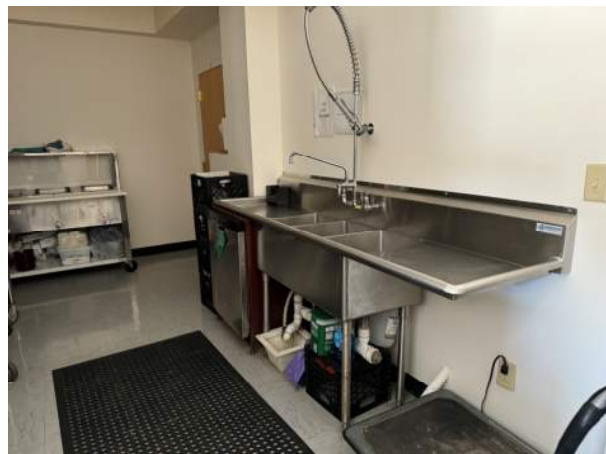
Kitchen—no dishwasher or grease trap observed
