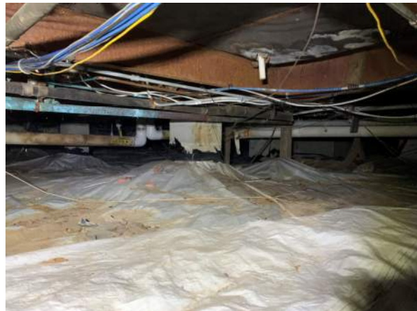
Corrosion of steel floor framing at crawl space
